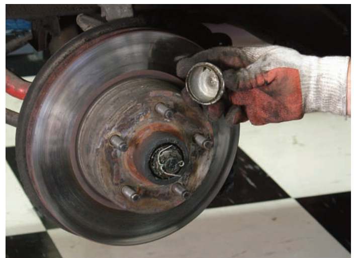
The dust cap was removed from the rotor so that the cotter key and spindle nut could be accessed. The cotter key was removed and the large spindle nut was disconnected with a large crescent wrench.
