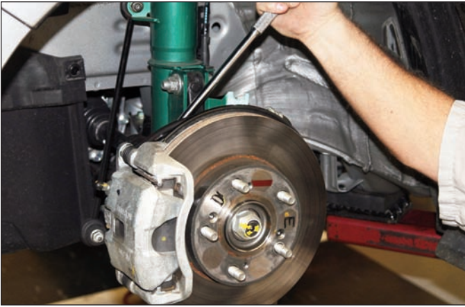
Sequence 7: Using a breaker bar and socket, break loose the caliper mounting bolts from the back side.
